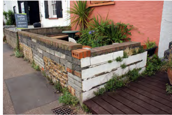
Poor boundary wall treatment
