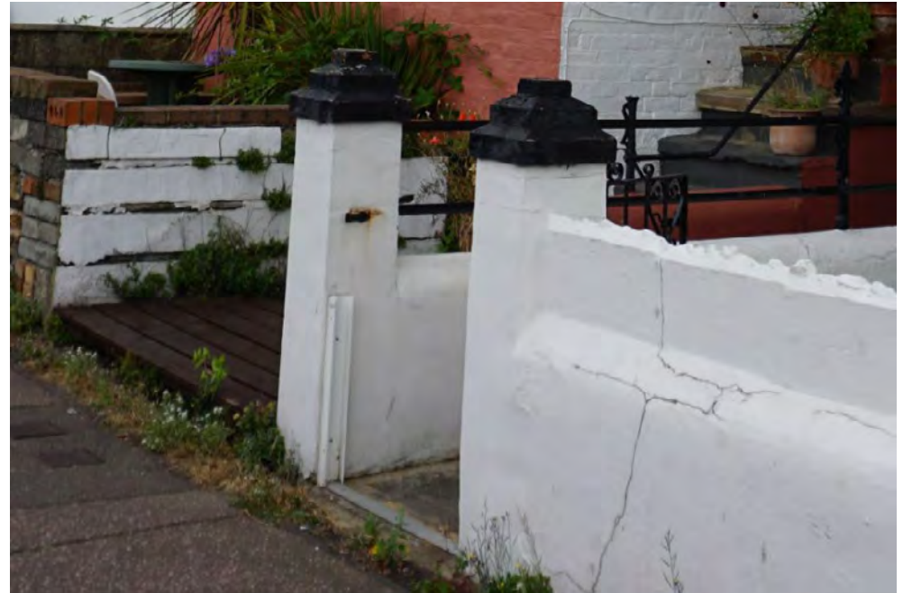
Aluminium rails for flood prevention barrier installed at the gate of No.46
