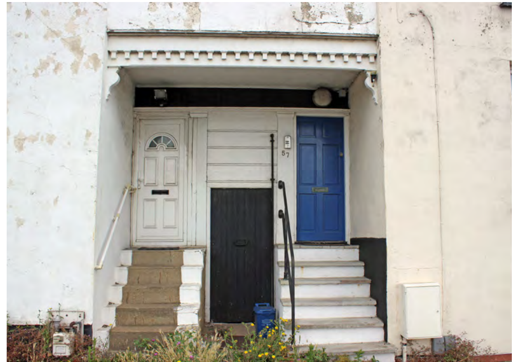
Replacement doors in 'off-the-peg' styles less appropriate to the character of the buildings
